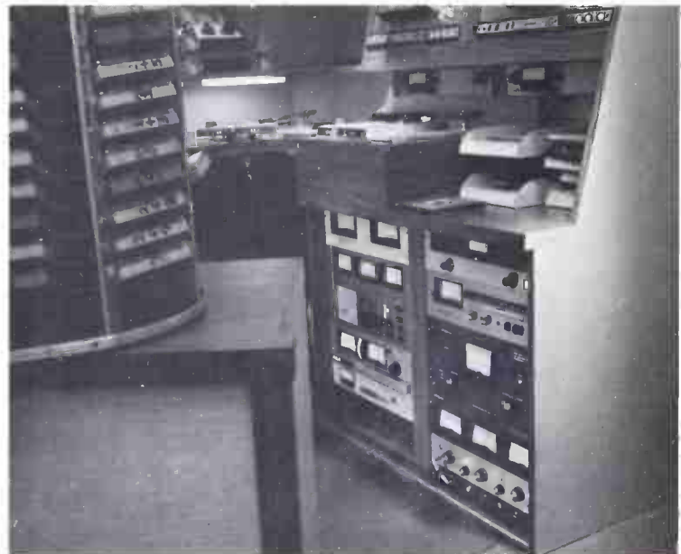
Control Console for the remote control of the AM and FM transmitter.
