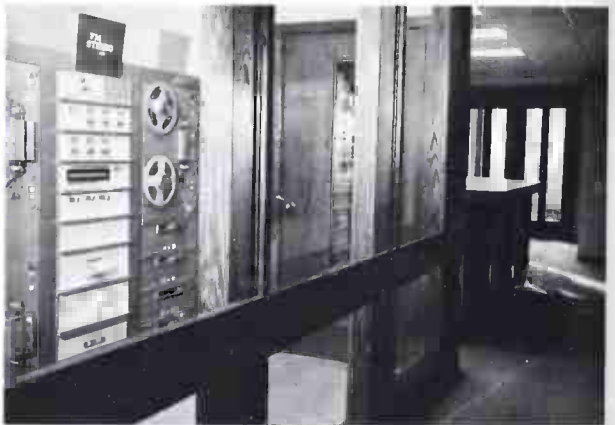
FM automation unit is on first floor in separate glassed-in room.
