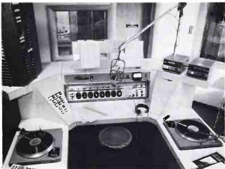
Closeup of WNHU control console. Pushbuttons on left sloping panel control Spotmaster carts, Revox and Scully tape recorders. Above Gates Yard Console is (right to left): annunciator panel which shows which studio doors are open, intercom controls, outside door lock control, EBS indicator, Right sloping panel has pushbuttons controlling telco lines.
