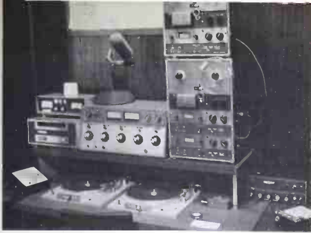
Photo of the compact WACI control facility.
