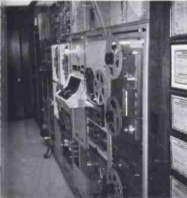
Looking down the passageway from the window in the control room.
